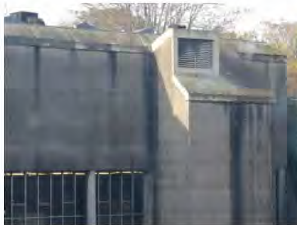
Staining on concrete facade
