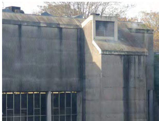
Staining on concrete facade
