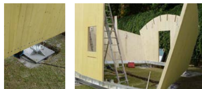
Picture 2: Walls anchored to foundations. Picture 3: Assembly of SWP on galvanised steel angled base plates (Photos: PRS Architects)
